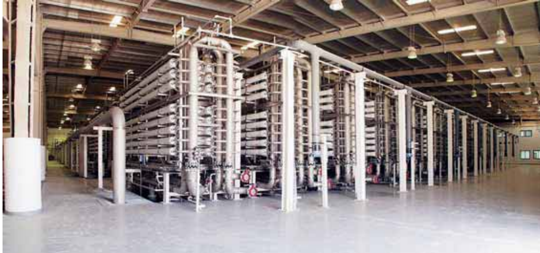
(8) Completed in 2004, the Sulaibiya Wastewater Treatment plant in Kuwait is one of the largest of its kind in the world (Source: Norit) [for high resolution version, see CD-rom]
